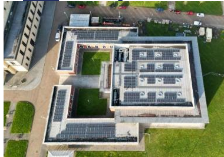
Bay Campus Library solar array
