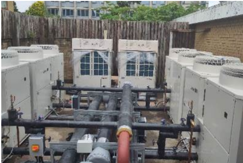
Haldane Building, air source heat pump
