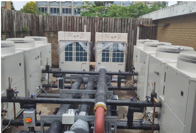
Haldane Building, air source heat pump
